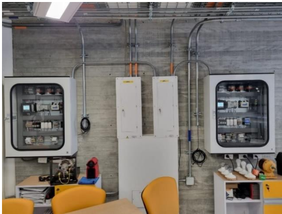
Figure 10. Finalized and operational panels. Source: own work.
