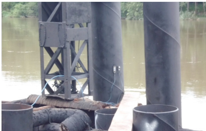
Figure 1. Example of installed accelerometer (right) and strain transducer (left) on the pile.
