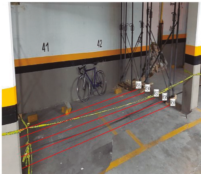
Figure 7. Location of the short profiles acquired in the basement at parking lots 41 - 42. Trajectories where profiles were taken are outlined in red. Note the great alteration in this parking lot, which shows a fairly large subsidence, as well as many cracks.
