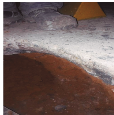
Figure 23. Evidence of scour. It is difficult to estimate the size of the scour, but it is seen to be elongated, which is consistent with what is observed in the GPR records. The exact position of the pit is unknown but is located at the foot of the retaining wall.
