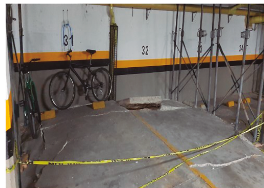
Figure 3. A rise is observed in the parking slab. The thickness of the slab is 15 cm. Several fissures and cracks have been formed.
