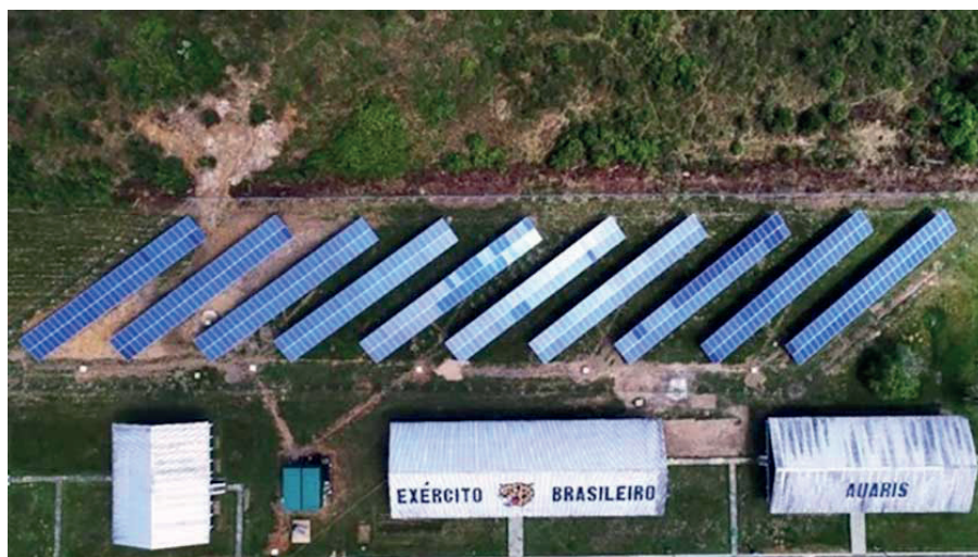
Figure 4. Photovoltaic plant at the 5th PEF (Auaris/RR)
