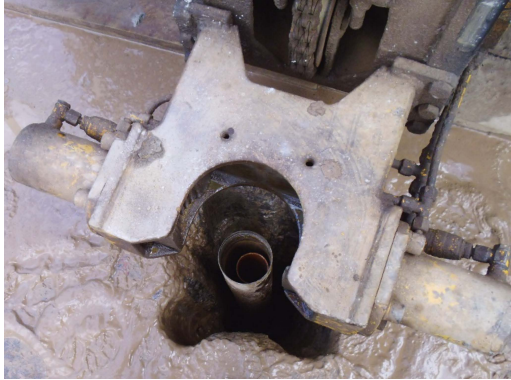
Figure 4. Piezometric space for groundwater level reading into borehole SE1-26. Source: IDU (2015b)
